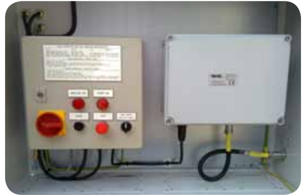
Main Control Panel pictured on the Left, Ignition Transformer pictured on the Right
