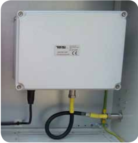
High Tension Generator
